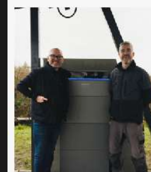
Robert McDonagh Futureproof Energy Installer in City, Texas
